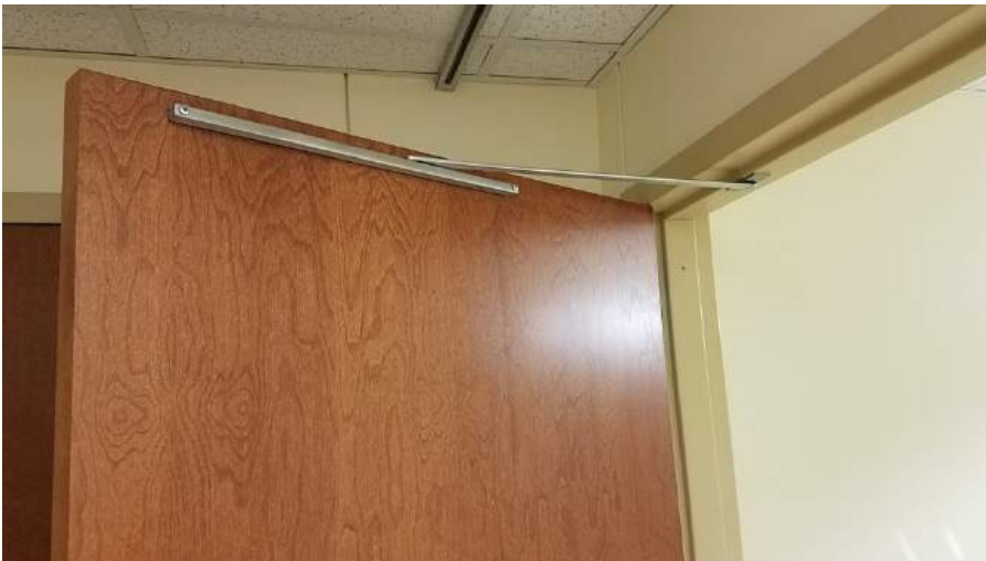
Overhead door stop.
