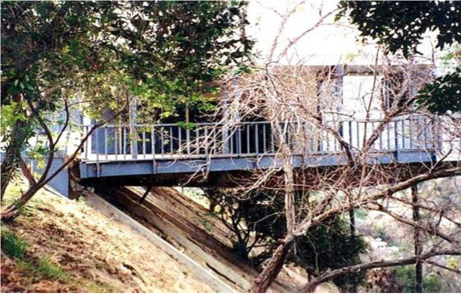
Figure 3. Hillside dwelling pulled away from uphill foundation in the 1994 Northridge, California Earthquake (Credit: City of Los Angeles Department of Building and Safety). Red arrow shows location where floor framing has pulled six to eight inches away from the uphill foundation.
