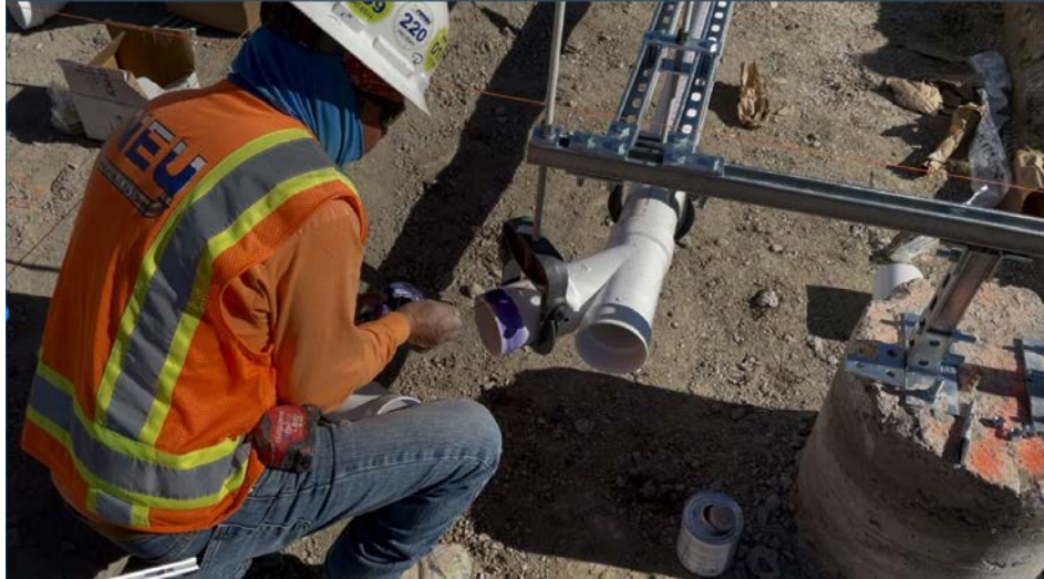
Photo: An example of a patent-pending construction method that allows installing plumbing under slabs-on-voidforms and provides complete isolation from expansive soil effects.
